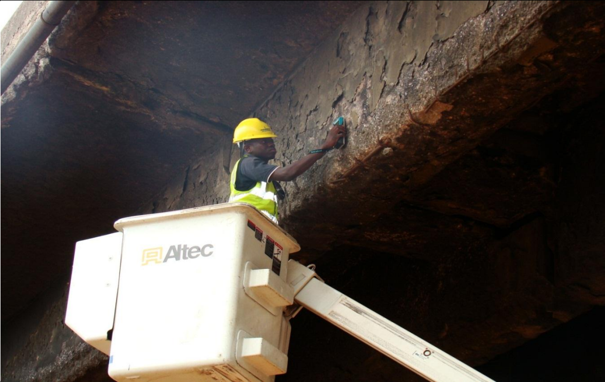
PLATE 3: ENGINEER TESTING FOR CONCRETE COVER AND BAR LOCATION/DIAMETER ON THE BURNT BEAMS
