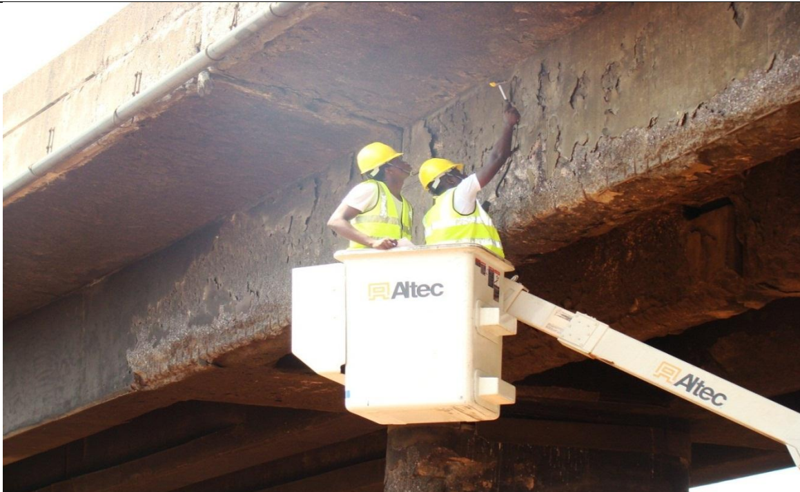
PLATE 4: SHOWING ENGINEERS TESTING THE BRIDGE BEAMS USING THE CONCRETE TESTER & SURVEYOR (CTS).
